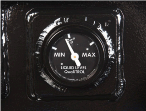
Main tank liquid level gauge
